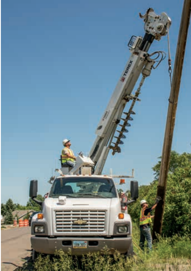
After the overhead conductor was removed, Journeyman Lineman Steve Kuball clamped the pole with a set of claws to control it. Journeyman Lineman Matt Hagen wrapped a cable from the winch around the pole, and the digger/derrick pulled the pole from the ground.
