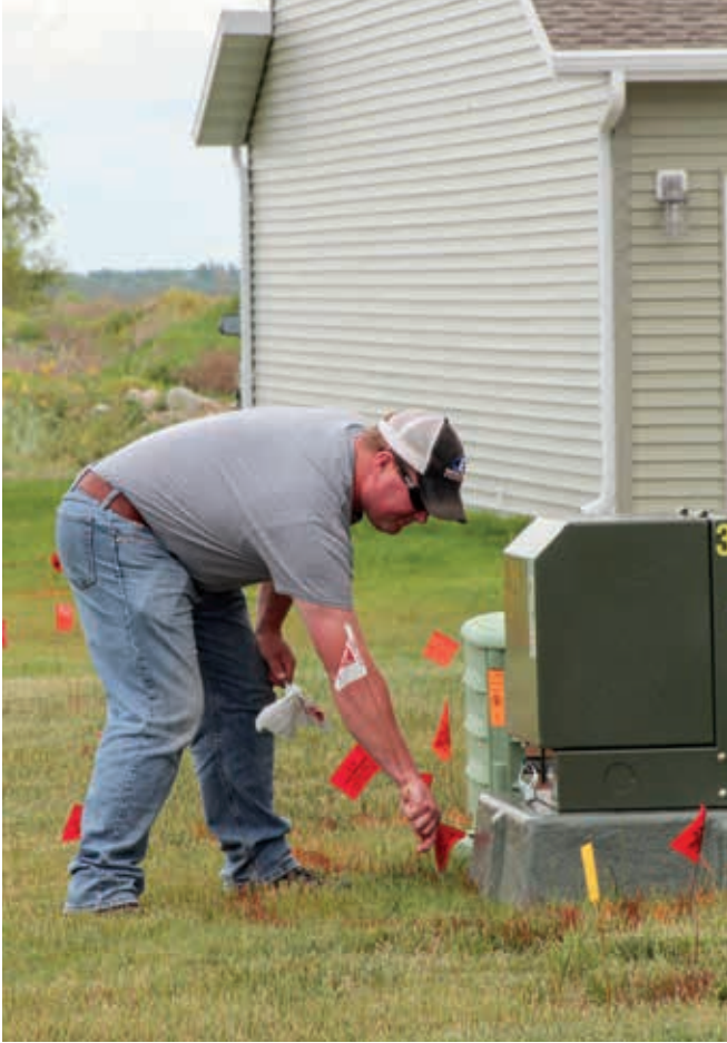
When converting from overhead to underground, the cooperative's staking department first plans the route in which to lay the cable. Here, Assistant Staking Engineer Beau Townsend shows how he places white flags in the ground to mark the route a contract crew will follow to trench or bore the powerline.
