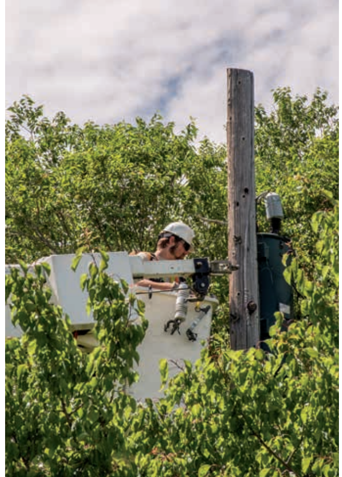
Capital Electric's linemen buried some overhead power line in housing developments adjacent to Washington Street. This will increase the system's reliability, because the mature trees will no longer be a threat to cause a power outage. Here, Journeyman Lineman Braden Martin prepares to retire the overhead line.
