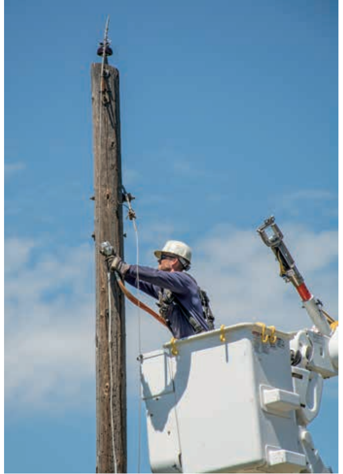
Once the linemen set and install the switches and terminate the cable, they energize the underground power line. Then, the overhead distribution line is ready to be de-energized and taken out of service. Here, Journeyman Lineman Lance Diebold cuts down the overhead line.
