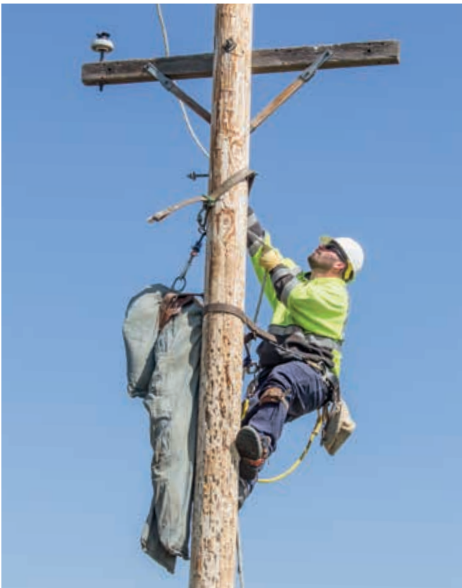
Charles Atkinson , lead lineman in Wing, throws his rope over the cross-arm in order to secure it, before threading it around the body of the mannequin.
