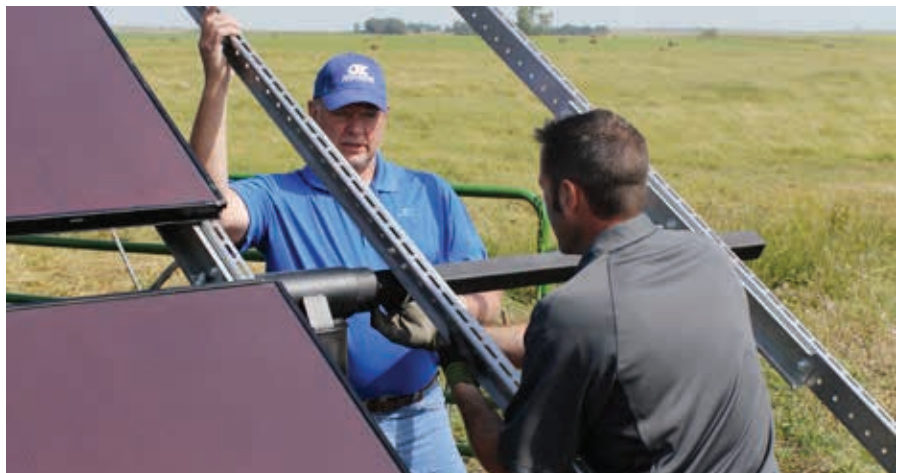
Doug Mork (left), member services director, says he’s worked on a lot of interesting projects with a lot of great people. Here, he helped Josh Schaffner , member services assistant, install solar panels next to a stock tank.
