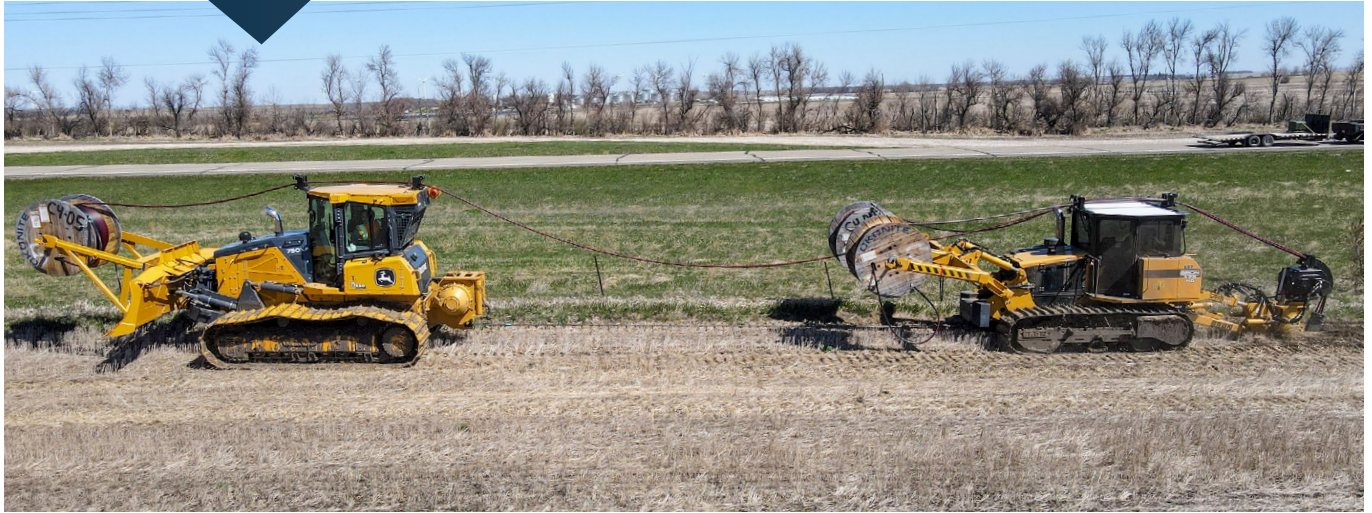
It's an efficient process to trench and bury underground cable with a plow train.
